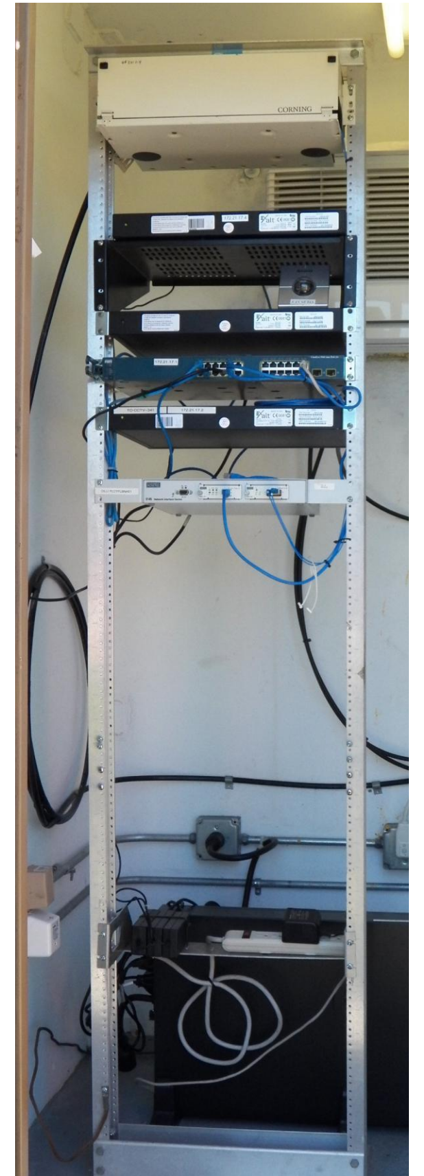
FLORIDA CITY HUB – ITS RACK
